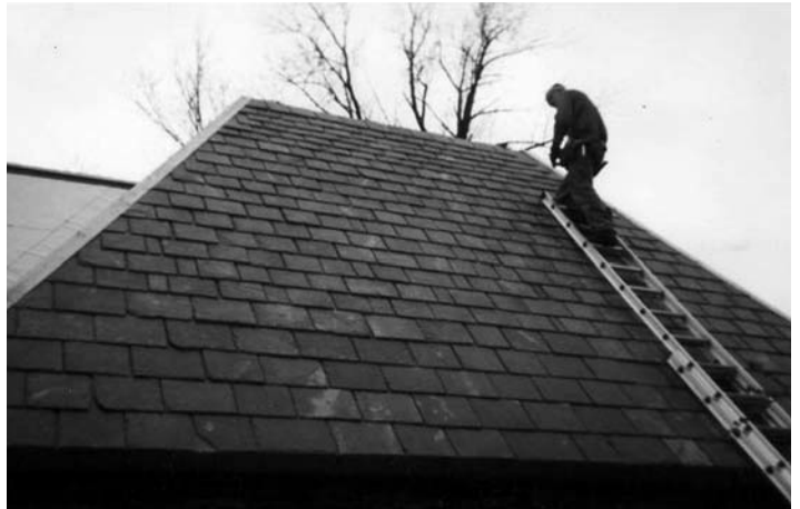
Putting the finishing touches on one side of garage, Erie, PA. Most of the faces had hips on both sides so we started in the middles and worked our way to the edges. Note how the steep roof pitch allowed us to lay ground ladders right on the roof, thereby avoiding the need for any roof planks.
