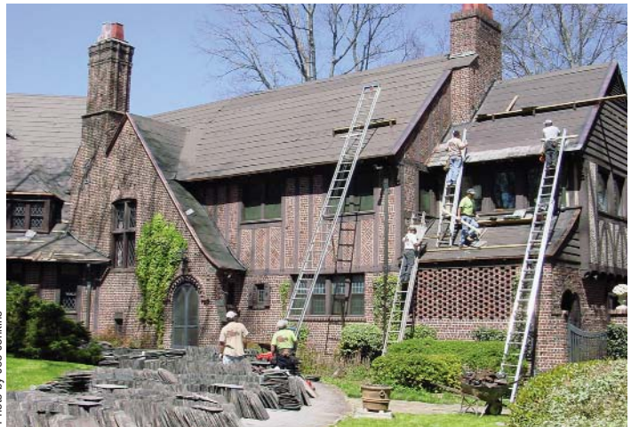
Glenridge Hall, front entrance, after the original slate had been removed and stacked in the driveway and the new felt installed. Re-slating is just beginning.
