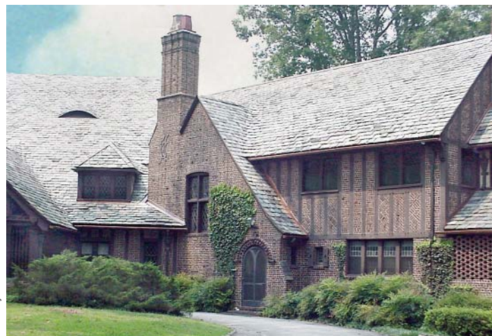
Glenridge Hall. The finished roof is not only beautiful, but also historically accurate. It can realistically last another century.
