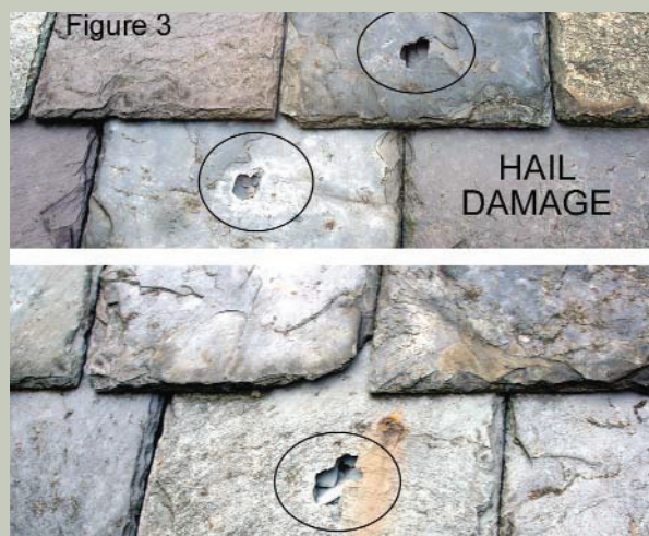
Figure 3 ▲ Hail-perforated slates should simply be removed and replaced. Hail damage is rarely a cause for the replacement of an entire slate roof.
