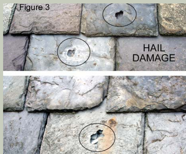
Figure 3 ▲ Hail-perforated slates should simply be removed and replaced. Hail damage is rarely a cause for the replacement of an entire slate roof.
