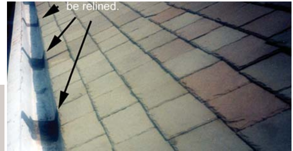
Figure 25 (above): Box gutters require expansion joints, otherwise the solder joints will crack under pressure. This is evident by solder joints that have been covered by roof cement, a common sight on box gutters, new and old.
