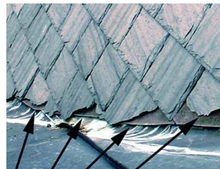
Figure 34: Slate roofing requires the correct tools to do the job right. There is no excuse for the sort of work shown above.
