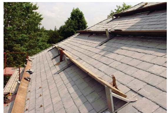
Figure 19: A correctly-staged slate roof will enable the roofers to install the slate without the need to walk on the shingles.
