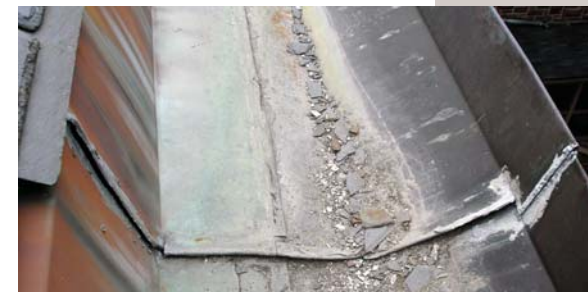
Figure 27: This is a perfect example of a new built-in gutter showing failed solder joints because not a single expansion joint was installed in the gutter system.
