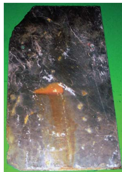
Figure 2: This Spanish black slate leached rust stains down the new slate roof after only one year.
