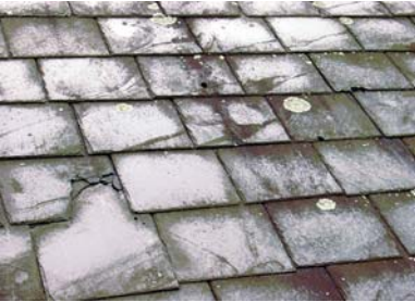
Figure 13 (above): Each course of slates should have been staggered so as to break the course below down the center. Instead, these slates were butted directly over the underlying slating nails, ensuring leakage.
