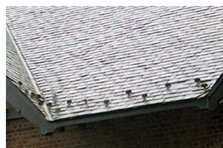
Figure 32: Snowguards must be installed in adequate quantities, or else they will get knocked off in the first bad ice storm and will damage the roof in the process.
