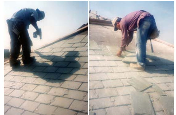
Figure 18: It is a mistake to walk on a slate roof during installation.
