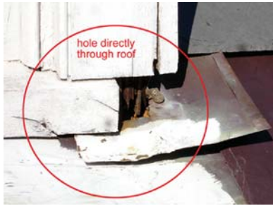
Figure 24 (above): This is a case where the corner flashing is neither folded nor soldered, leaving a large hole in the roof.
