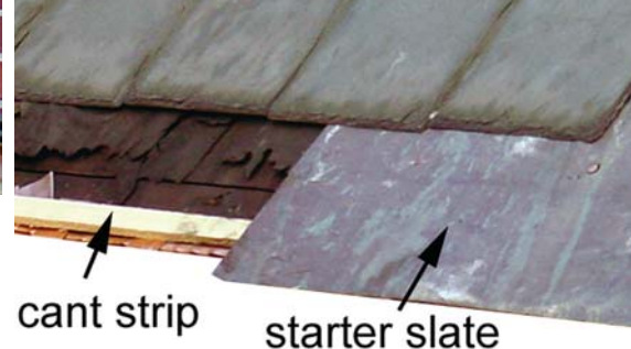
Figure 7 (above): Note that the starter slate is laid back-side-up and is propped up by a cant strip.
