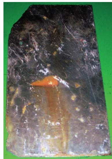
Figure 2: This Spanish black slate leached rust stains down the new slate roof after only one year.
