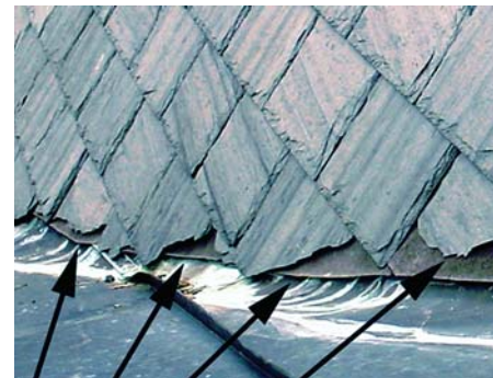
Figure 34: Slate roofing requires the correct tools to do the job right. There is no excuse for the sort of work shown above.
