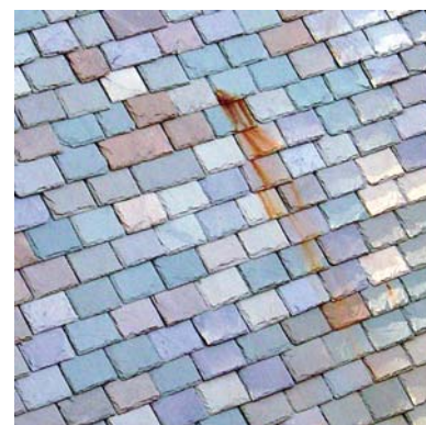
Figure 3: Even domestic slates can rust. These Vermont slates on a high-rise apartment were poor in quality and should have been screened for pyrite inclusions.
