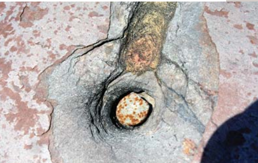
Figure 15: A protruding nail head eventually wears a hole in the overlying slate.
