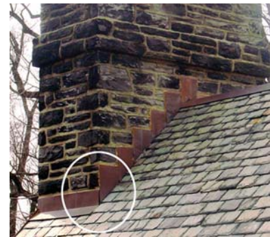
Figure 22 (above): Chimney corners flashings should either be folded or soldered. If neither is evident, then the corner is either sealed with sealant, or with nothing. In either case, this is a leak waiting to happen.
