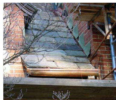
Figure 31: This gutter is just waiting for a snow avalanche to knock it off.
