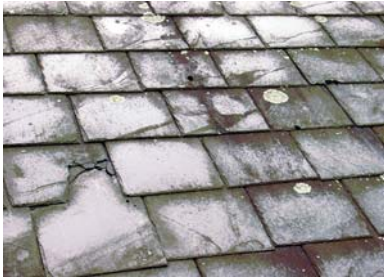
Figure 13 (above): Each course of slates should have been staggered so as to break the course below down the center. Instead, these slates were butted directly over the underlying slating nails, ensuring leakage.
