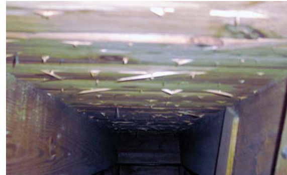
Figure 17: When the slating nails are too long, the back of the roof decking breaks out. This reduces the effective holding power of the nail. A longer nail, therefore, does not mean more holding power. The best nail length just barely penetrates the roof deck, if it penetrates at all.
