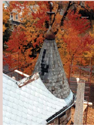
Crookston's Upright, Inc. constructs a new conical roof (top) and restores an old one with slate (above).
