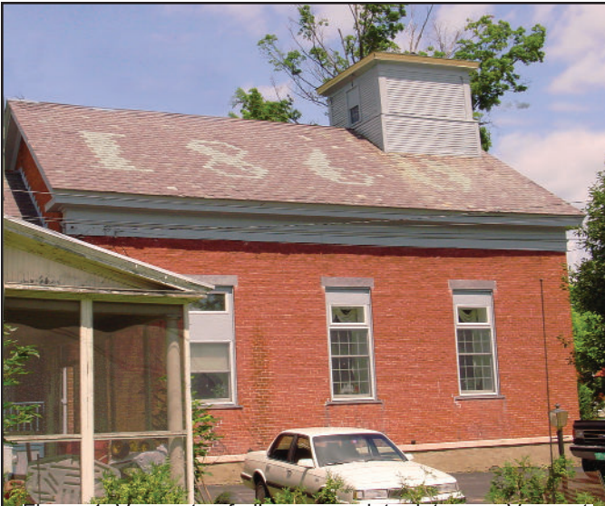
Figure 1: Vermont unfading green slate date on a Vermont purple slate background, photographed in 2003 at 143 years of age and still going strong.
