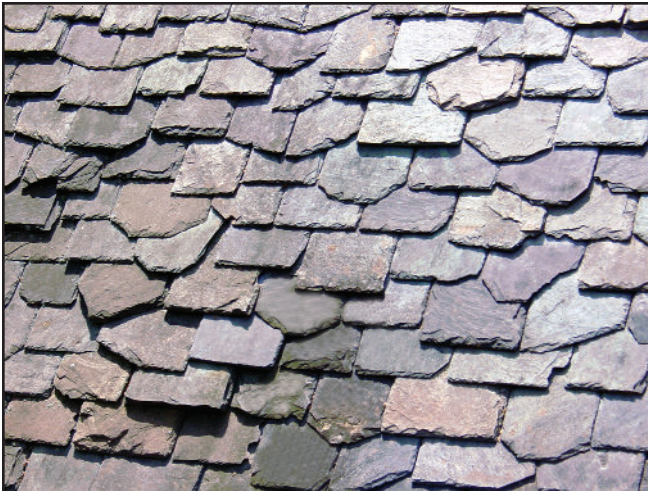
Figure 8: Ragged butt slate roof. Slates vary in widths, and lengths, and, in this case, colors. The top of the slates are lined up, but the bottom is allowed to hang down like a staggered butt roof, but the bottom edges are trimmed at random to create a unique look.
