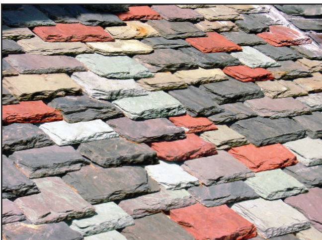
Figure 7: Staggered butt slate roof. Slates vary in widths, and lengths, and, in this case, colors and thicknesses. The top of the slates are lined up but the bottom is allowed to hang down.
